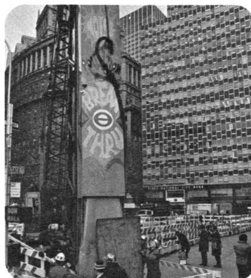
2. Pile cap nears ground level, where driving is more difficult and impact noise is closer to people in the immediate area. Bottom "skirt" is a flexible Kinetics type KNC Noise Control Curtain barrier that reduces noise by shielding the point of impact.
