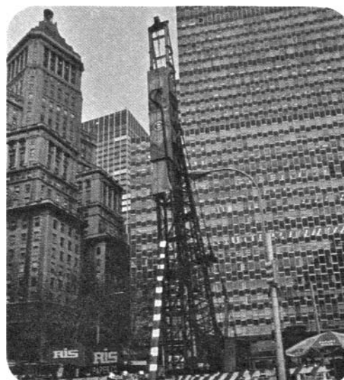
1. Colorfully decorated steel enclosure, with an "E" for Ecology on the outside and Kinetics composite noise absorption material bonded to the inside, surrounds pile driver and shock-treated pile cap. Web and flanges of pile have bands of Kinetics type KDC-E-162 viscoelastic damping compound applied to them.
