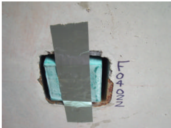
Figure 1: The fiberglass pad inserted in the encased mount, in the underside of the floating slab was secured temporarily with metal tape.
